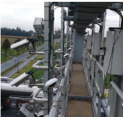
SEPTENTRIO GNSS antenna placement on highway gantry.
